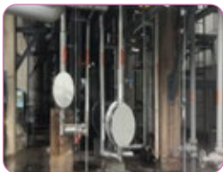
Clear labeling of pipeline contents and flow directions
