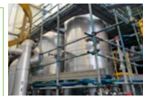
Gas-liquid separators at the front end of control equipment
